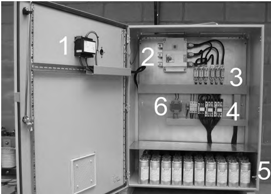
Figure 3.10 – Automated power factor correcting capacitor bank.
